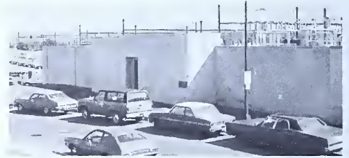
Capitol Complex Substation.
